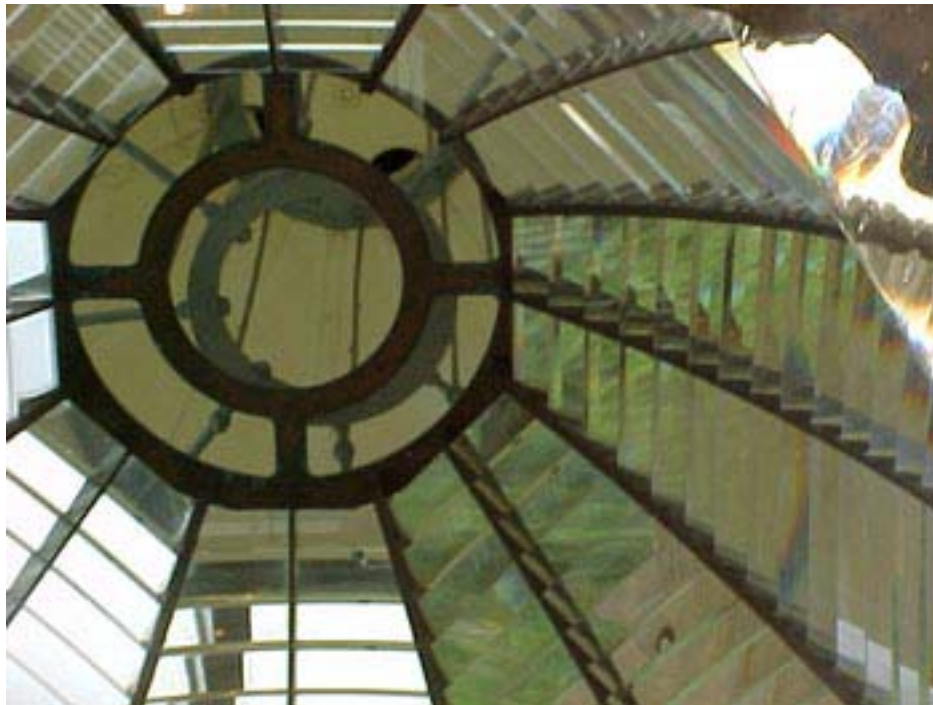
Figure 3-3. Out of Plumb
