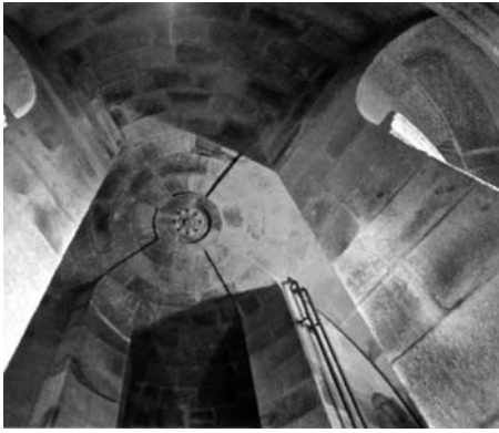
The interior of the tower. Photo from The World's Greatest Lighthouses by Annamaria "Lilla" Mariotti.
