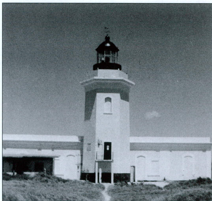
Above – Cape Rojo lighthouse as it appears today. The windows have been blocked and due to its remote location it has not been heavily vandalized. Photo by District Inspector Gris Boxley.
