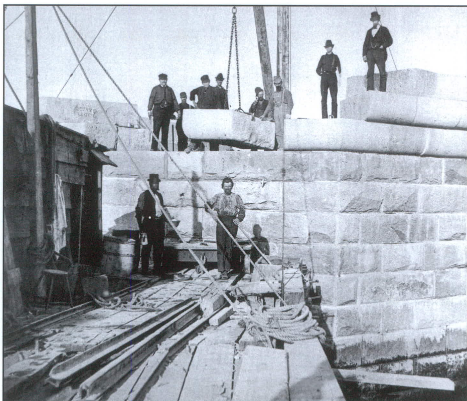
Lifting a foundation stone from the work barge to the foundation, 1873. National Archives photo.
