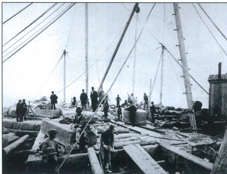
Working on Race Rock in 1873. The work barge is in the foreground. Surveyors can be seen on the edge of the foundation at left. The poles are various cranes mentioned in the article. National Archives photo.
