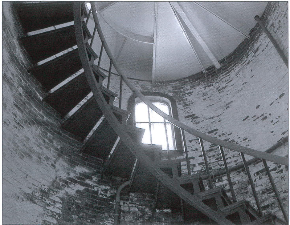
Interior view of Cape Neddick Lighthouse. The cast iron exterior is lined with brick and has a cast iron stairway. Photo by Jeremy D'Entremont.
