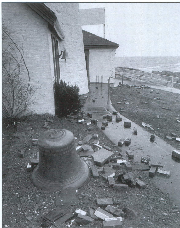
Destruction at the Portland Head Light Station from a similar storm in 1975. Base of tower at left, fog signal building upper middle. Note the fog bell torn from its base. U. S. Lighthouse Society photo.
