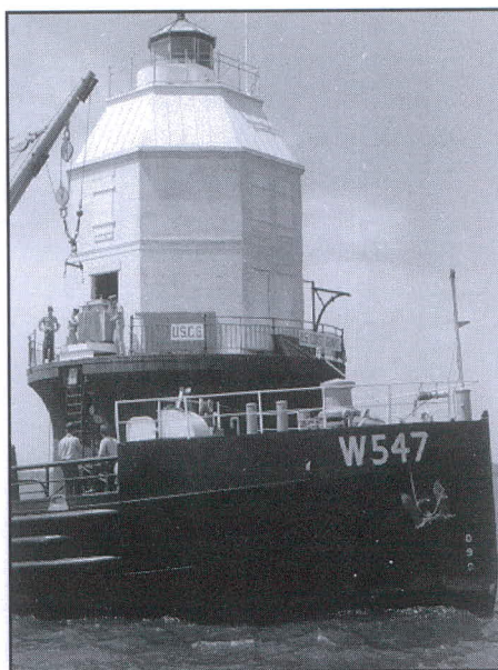
U.S. Coast Guard Cutter White Pine at the Baltimore Lighthouse installing the Nuclear Generator. Photo courtesy of the Coast Guard historian's office.
